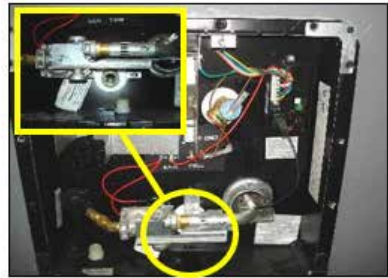
Fig 1: Water Heater Drain Plug
