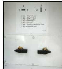
Fig. A - Water Valve Controls
