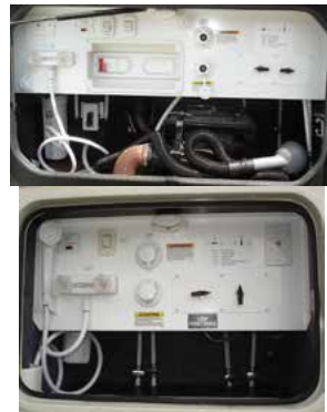
Fig. B - Utility Center
