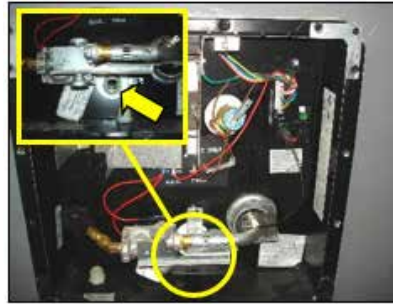
Water heater drain plug
