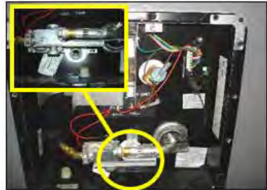
Fig 1: Water Heater Drain Plug
