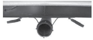
Black/Grey Tank Drain and Valves
