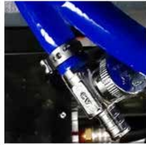
Fresh water drain valve
