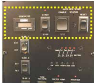
Command Center Panel
