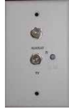
Antenna Power Supply
