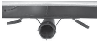
Black/Grey Tank Drain and Valves
