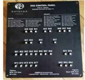
GFCI Breaker Panel
