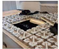
Water heater Bypass
