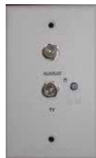
Antenna Power Supply
