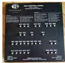
GFCI Breaker Panel
