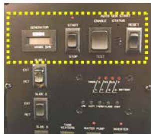
Command Center Panel
