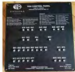
GFCI Breaker Panel
