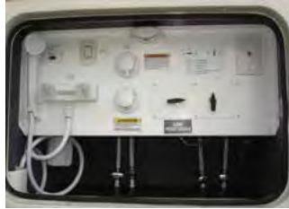
Fig. B - Utility Center
