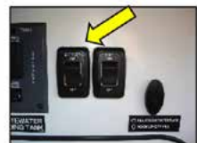
Macerator power switch
