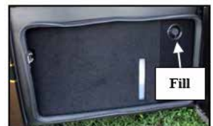
Fresh Water Tank
