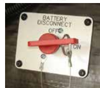
Battery Disconnect Switches
