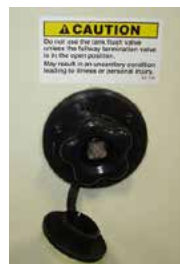
Tank Flush Inlet
